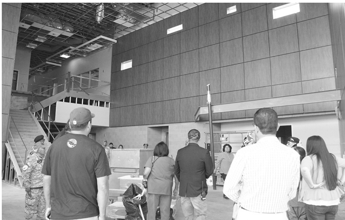
Councilman Devin Redbird leads a tour group through the spacious front lobby of the future, two-story District 7 Service Center.
