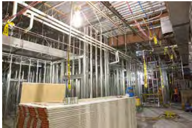
Exposed steel beams and wires can be seen inside the old primary care facility as crews work hard to complete the renovation.
