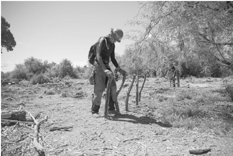
A DEQ Fuels Crew members prepares posts for an artificial beaver dam under construction. Christopher Lomahquahu/GRIN
