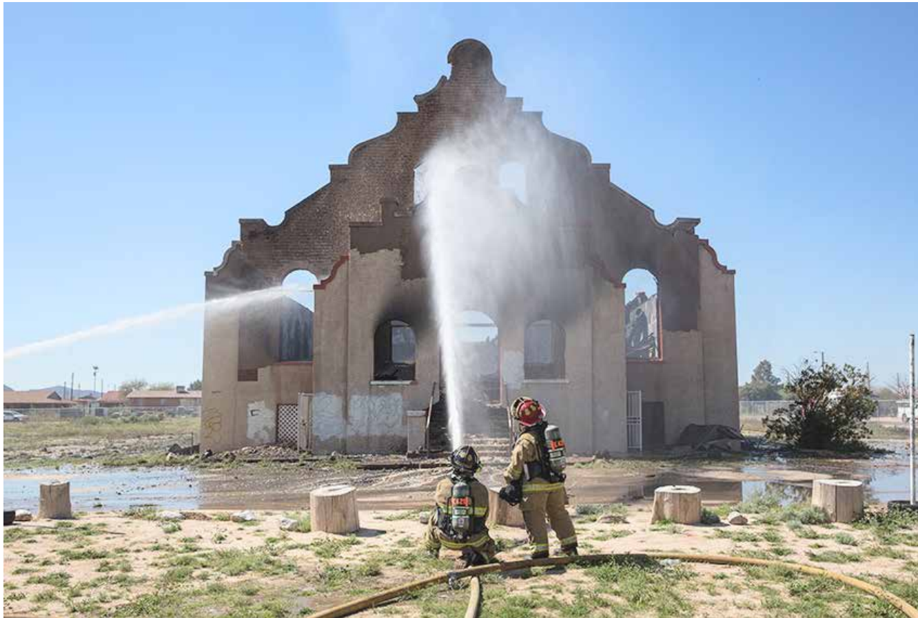
Crews put out the fire at the historic Presbyterian Church in Sacaton on March 25. Christopher Lomahquahu/GRIN
