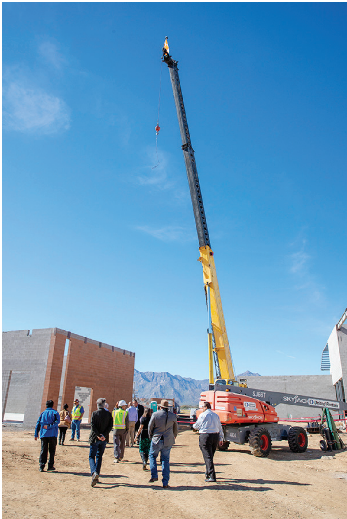
The Gila Crossing School Construction Owner's Team walks along the main corridor of the future school on Jan. 24 in District 6. Roberto A. Jackson/GRIN
