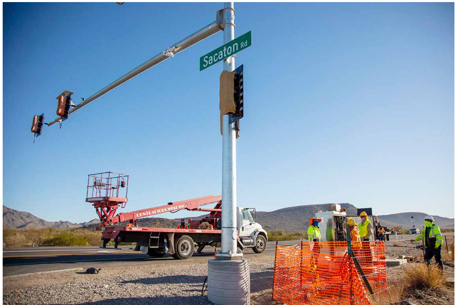
Crews work on the new stop light at Sacaton Road and SR87 on Dec. 2. Emma Hughes/GRIN
