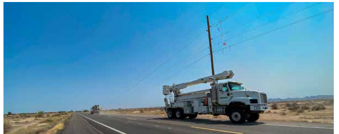
GRICUA crews work to repair damaged power lines along Highway 587 in District 5. Kyle Knox/CPAO
