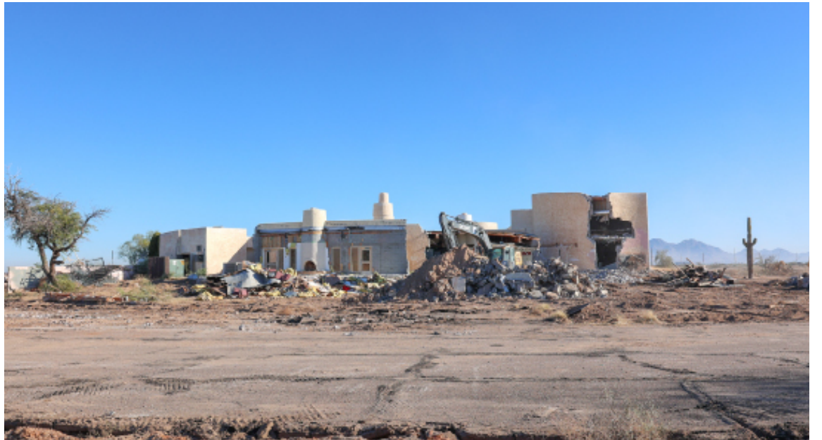
Demolition of the Arts & Crafts building, located off the I-10 and Casa Blanca Road, is the beginning of future development for the 40 acre lot. Emma Hughes/GRIN.
