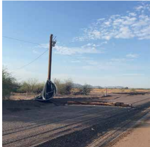
A damaged power line, along the 587 highway, after a catastrophic monsoon storm in July 2021. Photo courtesy of OEM
