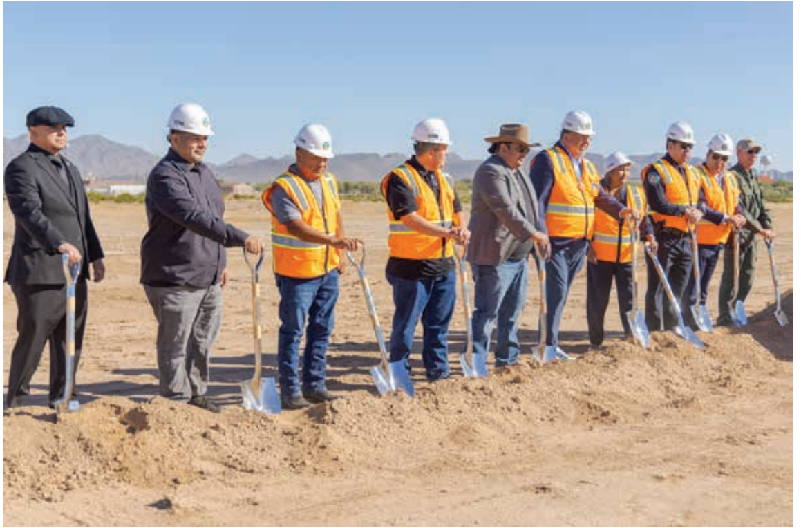
Members of the GRIC Community Council, Gov. Lewis, Lt. Gov. Monica Antone, and GRPD at the ground breaking for the new GRPD police department building in Sacaton. Kyle Knox/GRIN
