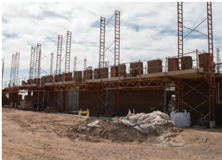
Ongoing construction of the support building for the Gila River Police Department facility that will hold the k-9 unit and Gang unit. Velia Moncada/GRIN
