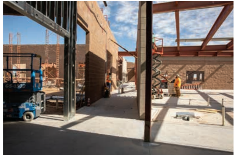
Hallway of the new Gila River Police Department facilities during construction, that will feature a calendar stick showcasing the GRPD law enforcement history. Velia Moncada/GRIN
