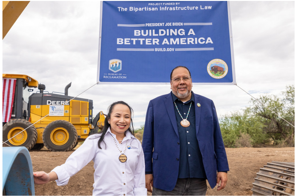
U.S. Bureau of Reclamation Commissioner Camille Touton and Gov. Stephen Roe Lewis stand at the construction site for the new 19-mile pipeline. Kyle Knox/GRIN
