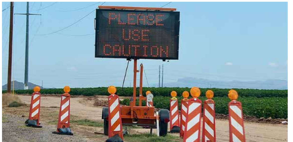
Sign reminds motorists to use caution while road work and construction takes place along State Route 87. Photo Courtesy of Joseph Morales
