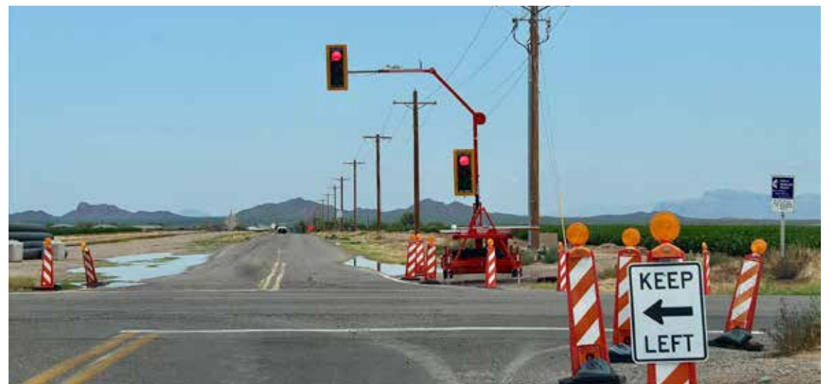
Temporary traffic signals have been placed at the intersection of State Route 87 & Skousen road. Photo Courtesy of Joseph Morales
