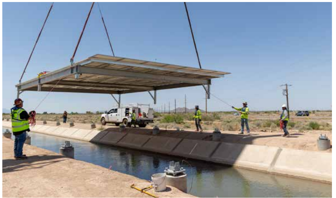
Solar panels are installed over the Casa Blanca Canal on May 22. Emma Hughes/GRIN
