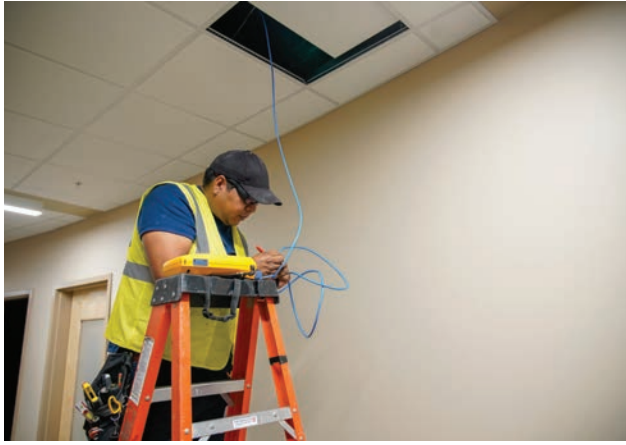
Wi-Fi installation at one of the District Service Centers. Photo Courtesy of Gila River Telecommunications Inc.
